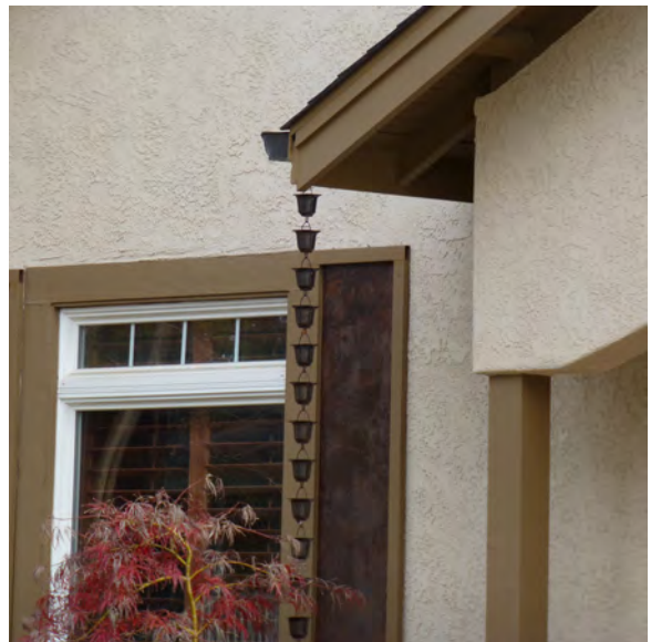
Rain Chain Connected to Gutter
