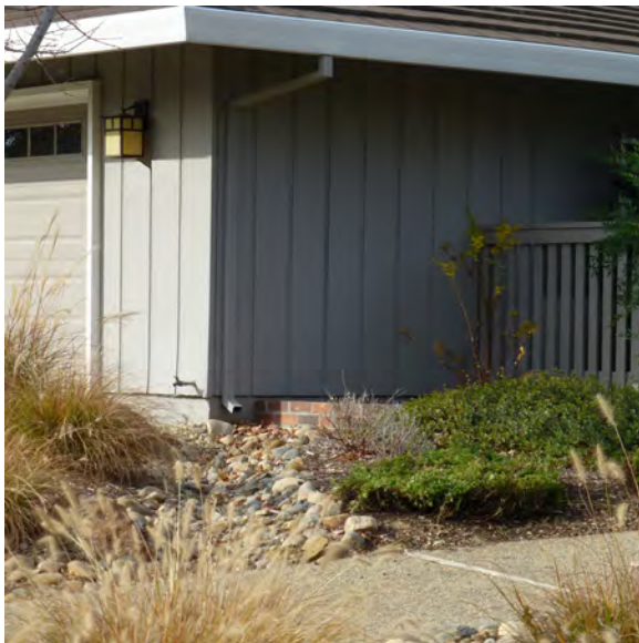
Downspout Connected to Gutter Directed to Dry Creek Bed
