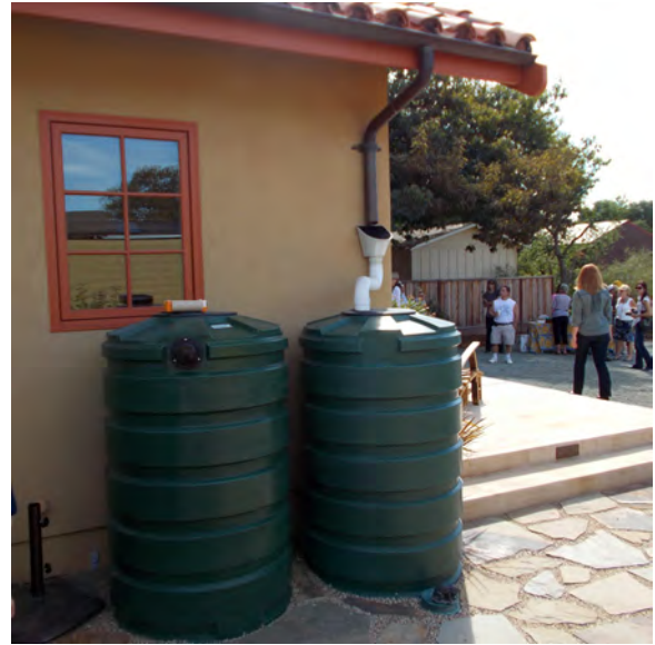
Downspout Directed to Rain Barrel
