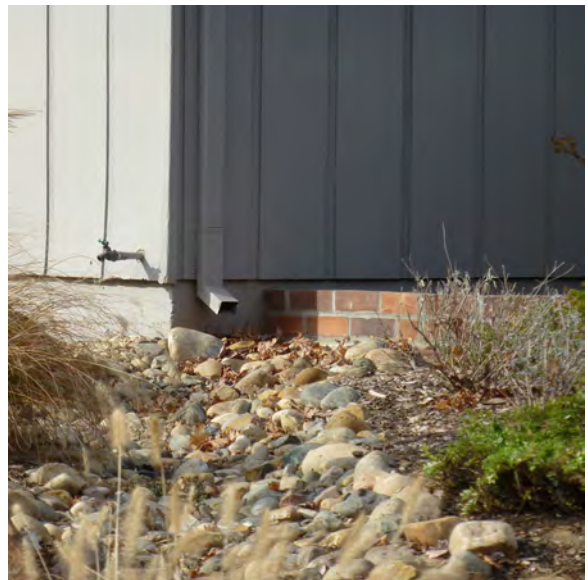
Downspout Directed to Dry Creek Bed
